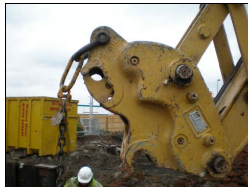
Figure 4 – Hitch tilted backwards with master link subject to twisting
